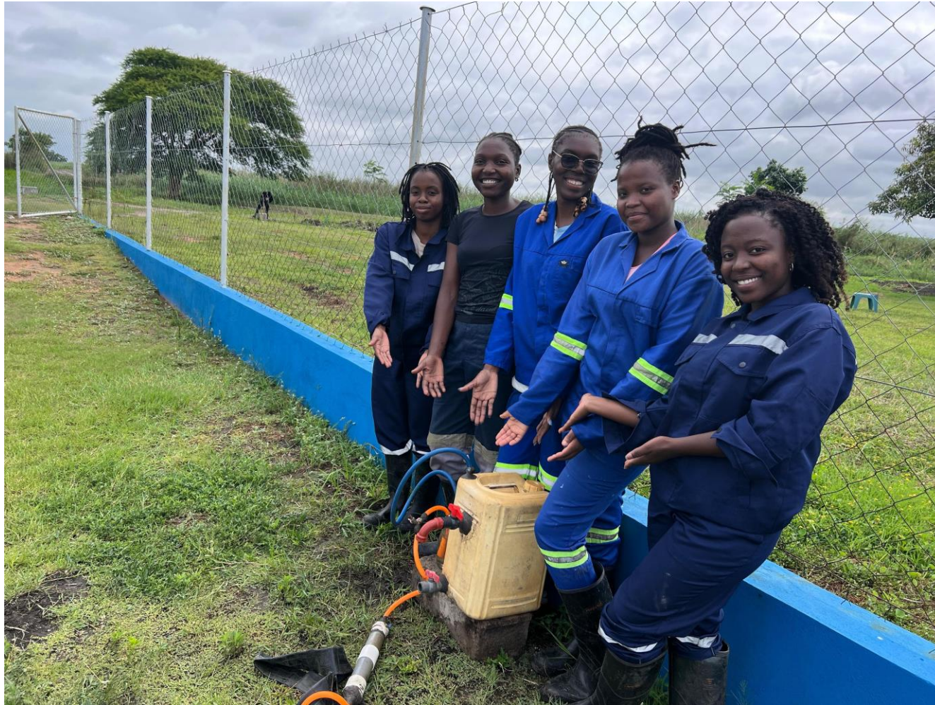
Photo: Happy End after the construction of the Biogester during the Girls' training.
