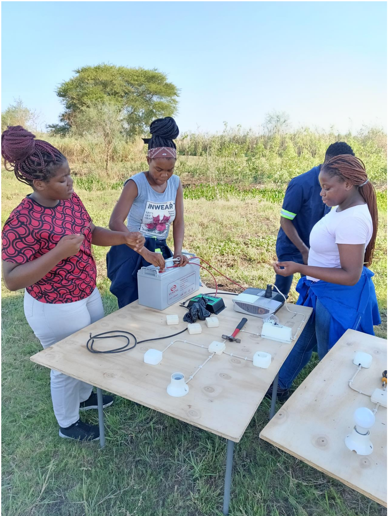
Photo: Trainees assembling a residential electrical installation and a photovoltaic system during a training course on the topic: Assembly and Operation of a Residential Electrical Installation and an Isolated Photovoltaic System.
